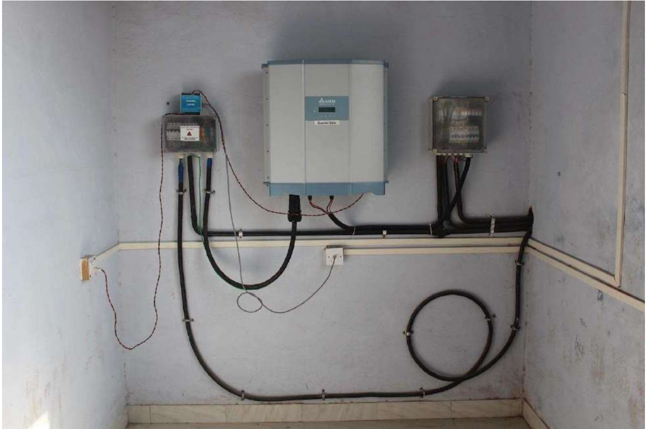
Solar On Grid System (Net-meter)
