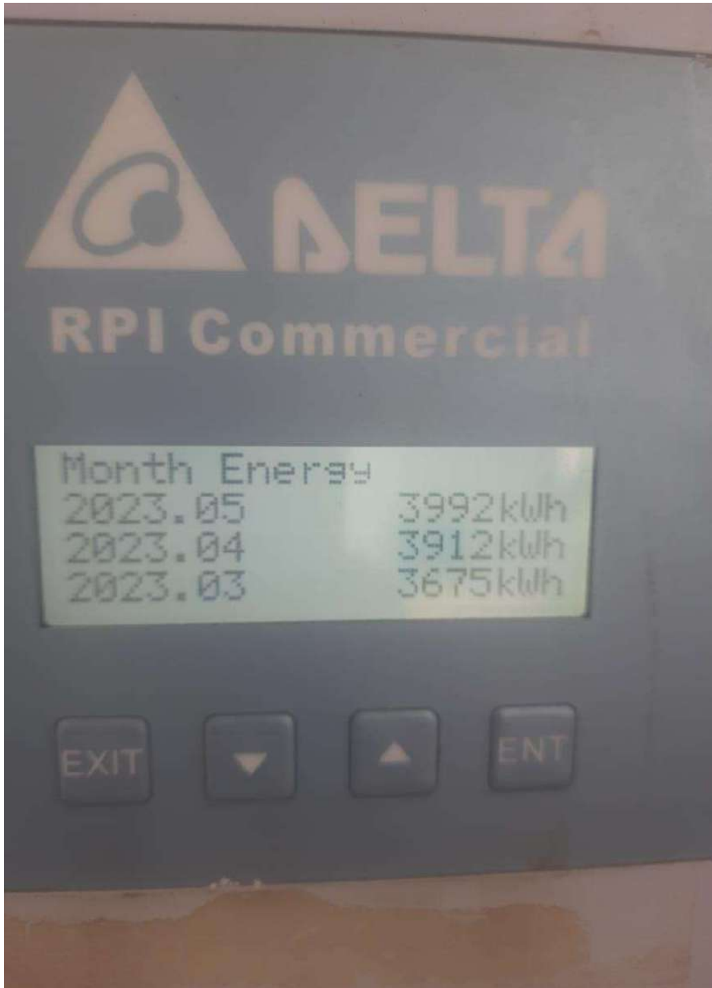
Meter Reading at Generation
