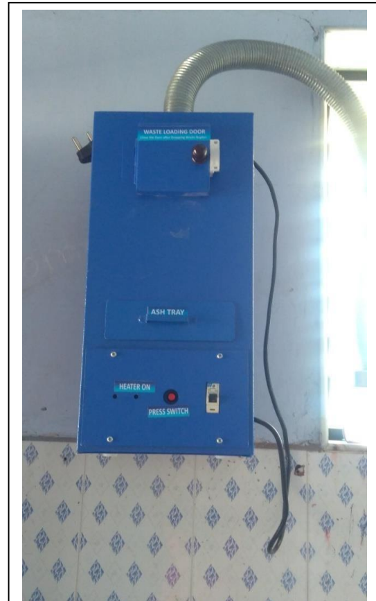
Incinerator in the Ladies washroom (main building )
